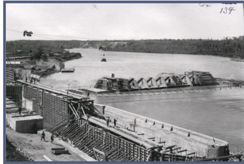
La Colle Falls Hydroelectric Dam Project, Photo Courtesy of Prince Albert Historical Society
