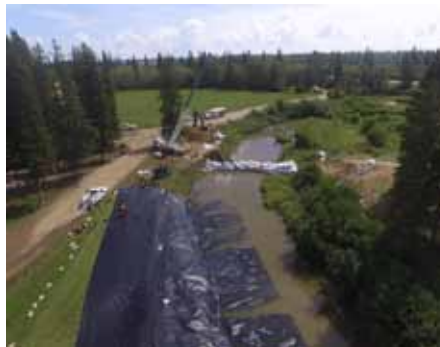
▲ Sandbagging at Little Red River Park to allow for water to be pumped to the Water Treatment Plant ▼
