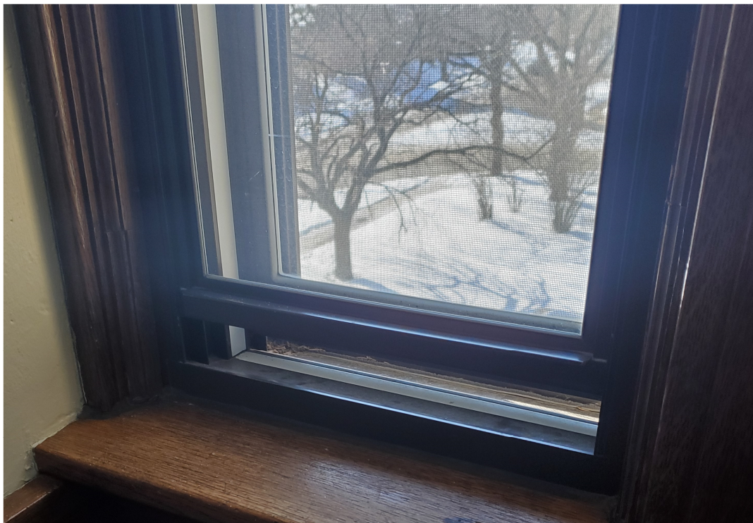
Figure 16 – Showing general configuration of the operable sash and frame – screen on exterior
