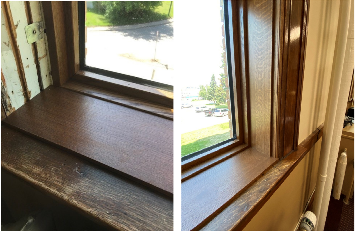
Figure 32 - 33 Detailing around new jambs and sill (original sill and casing – original frame has been left in place)
